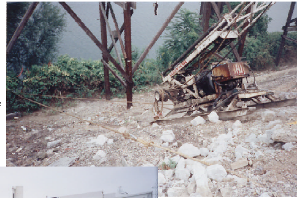
Right: Lowering of a drilling rig over a steep embankment to the Kanawha River's edge prior to monitoring well installation.
